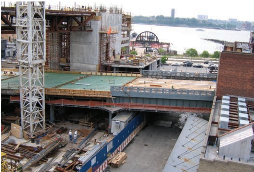
Enhancing the lower West Side of Manhattan, the Highline Greenway Park is being constructed on an abandoned elevated rail viaduct. This community project is managed by Friends of the Highline with many public and private partners.
