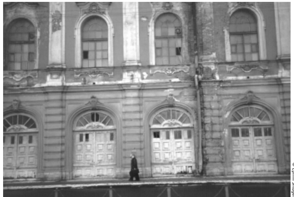
These former imperial stables are now dilapidated and occupied by auto repair workshops.
