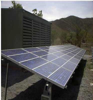
Figure 8: Photovoltaic Array (Arup)
