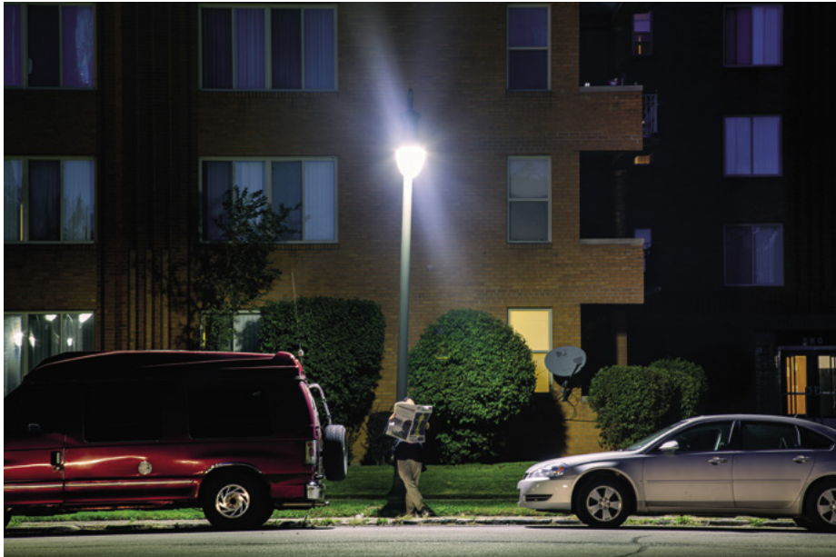
The installation of 65,000 network-enabled LED lights in Detroit brought many city blocks back from total darkness. Credit: Haomin Wei/Detroit PLA.
