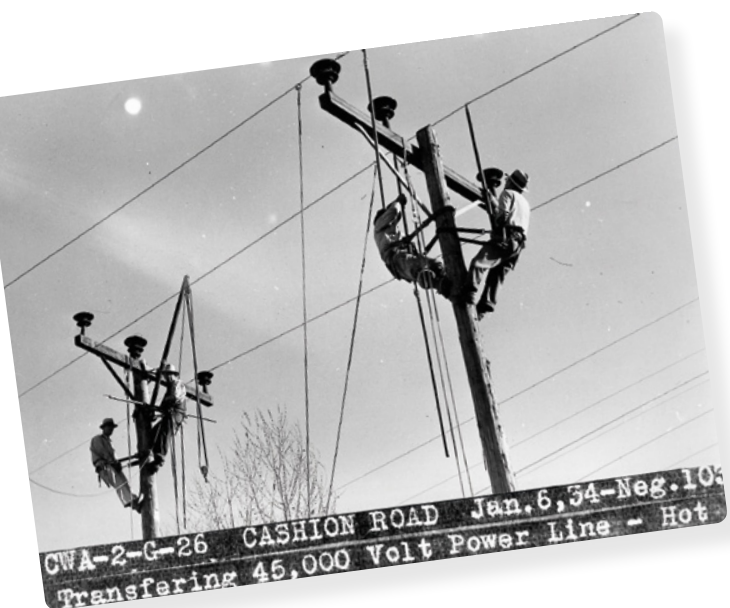
Construction of power lines in the Maricopa County town of Cashion, Arizona, in 1934. Credit: Arizona State Library, Archives and Public Records, History and Archives Division, Phoenix, #98-3250.
