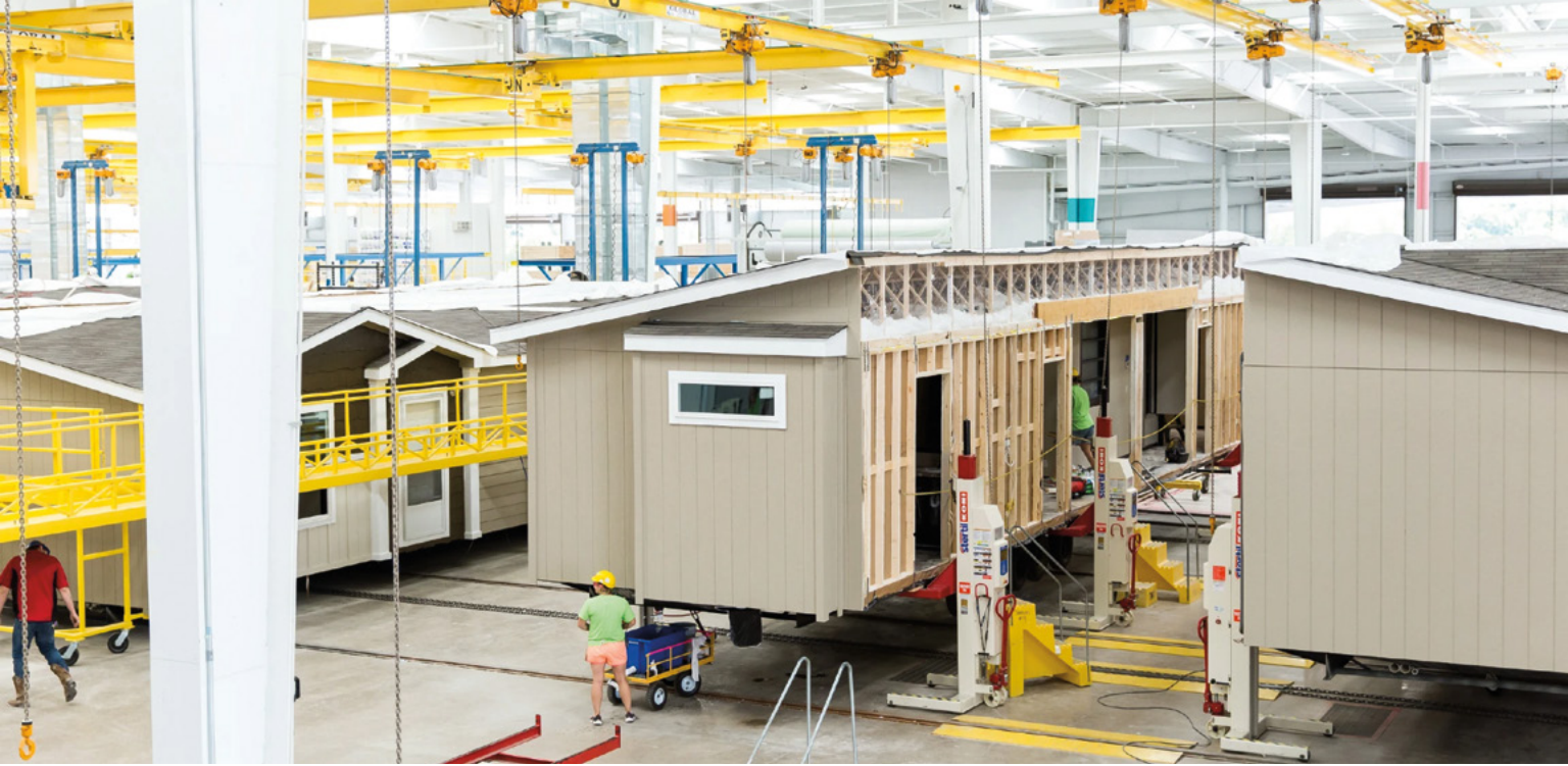
Manufactured homes under construction in a factory in Athens, Alabama. Credit: Clayton Homes.
