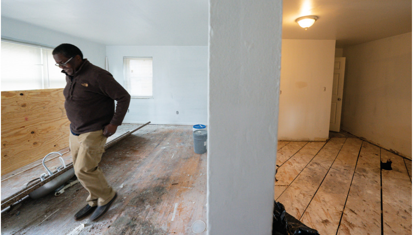
A contractor hired by the Port examines the condition of one of the agency's newly purchased houses. Credit: Jeff Dean.
