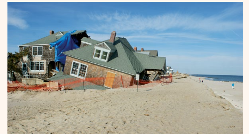
Hurricane Sandy damaged many homes along the New Jersey shore after making landfall there on October 29, 2012. Source: L. Johnson (2013).
