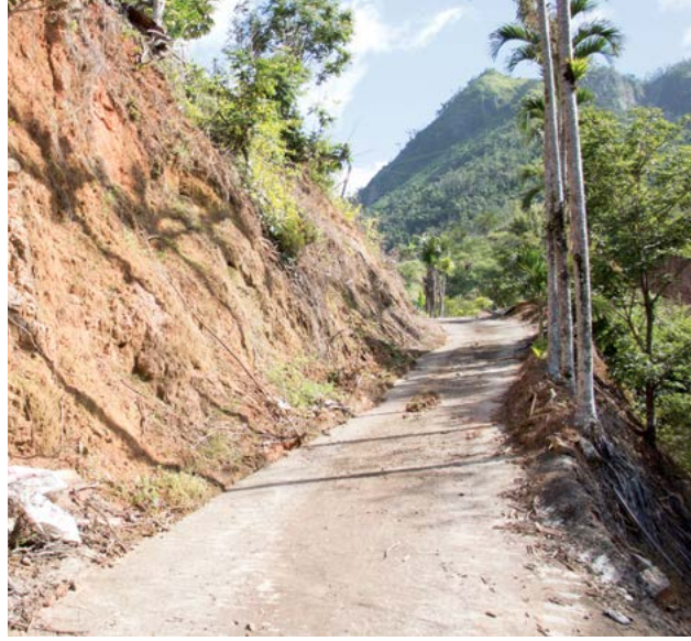
Many of the roads in Utuado were destroyed by Hurricane Maria, and incomplete repairs created hazardous driving conditions. Credit: Laura Galarza/Montclair State University
