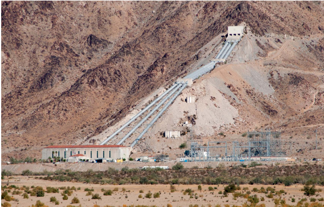
A California pumping plant sends Colorado River water uphill on its long journey to Los Angeles. Credit: NNehring via iStock.
