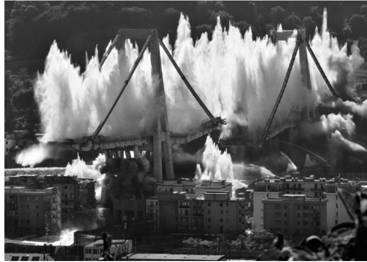
Demolition of the Ponte Morandi in Genoa, Italy, in 2019. One year earlier, a section of the bridge had collapsed. Credit: Gianluca Cichellero via iStock/Getty Images Plus.
