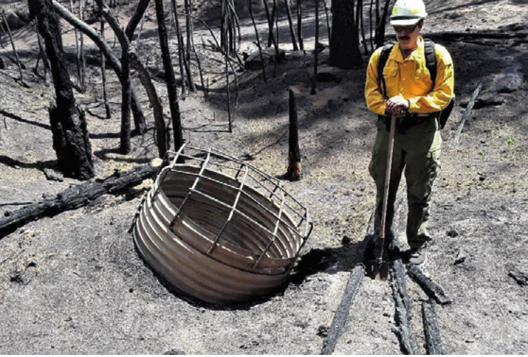
A soil scientist from the federal Burned Area Emergency Response (BAER) team inspects a culvert in the Hermits Peak–Calf Canyon burn scar in June 2022. Credit: U.S. Forest Service.
