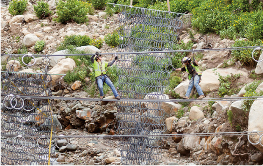
In 2019, workers installed steel mesh netting in San Ysidro Canyon above Montecito, California, to reduce the impact of post-wildfire debris flows. Two years earlier, mudslides had killed 23 residents of the community and destroyed 130 homes. Credit: Christy Gutzeit.
